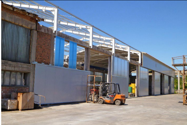
Expansion of the production site and large-scale restoration work on the ARJES premises in 2009 - 2011
